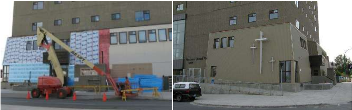
Before (left) and after photos of the Northern United Place retrofit this summer.
