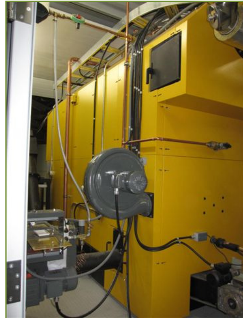
Wood Pellet Boiler at Chief Jimmy Bruneau School
