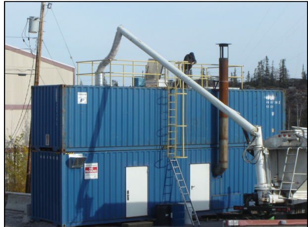
Commercial Pellet Boiler at Bison Apartments
