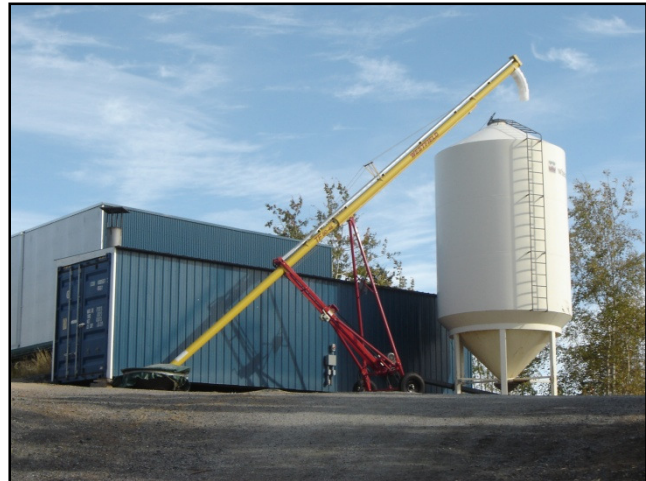
Commercial Pellet Boiler at Sir John Franklin
