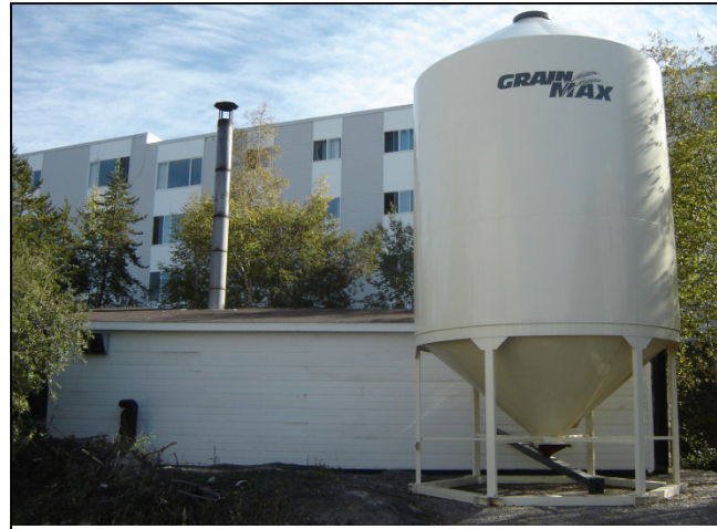
Commercial Pellet Boiler at Ft. Gary & Ridgeview Apartments
