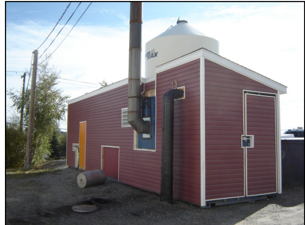
Commercial Pellet Boiler at Garden Townhomes
