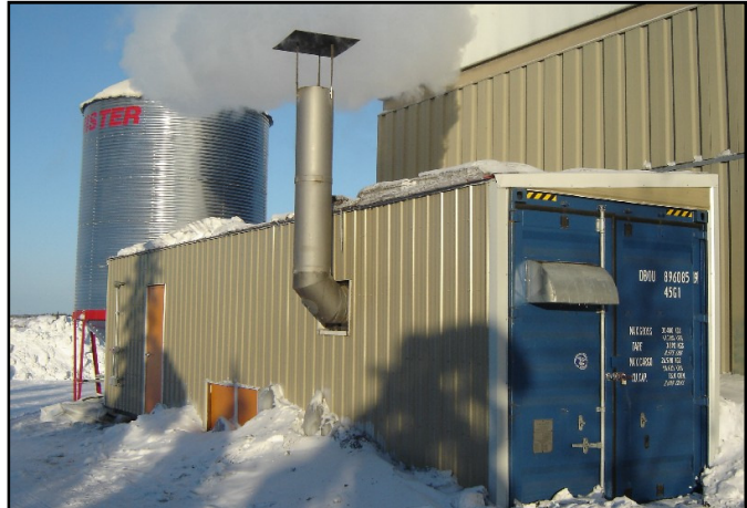
Commercial Wood Pellet Boiler behind YK Arena
